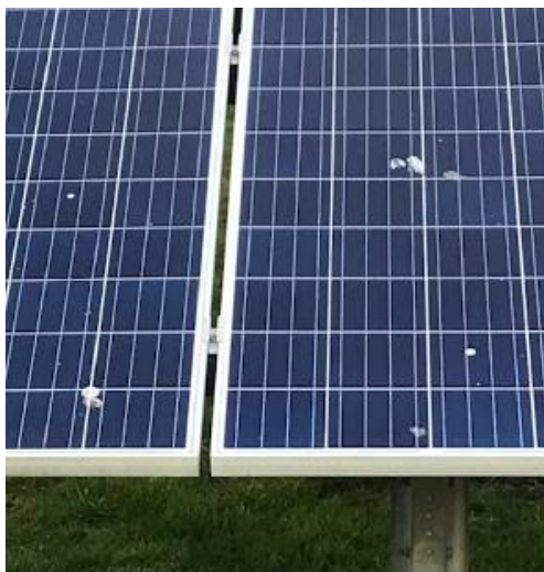
Figure 8: Gaps between panels at Partridge Farm solar farm
